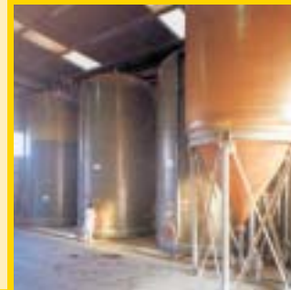
HAZARDOUS AND NON HAZARDOUS LIQUID WASTE TREATMENT
